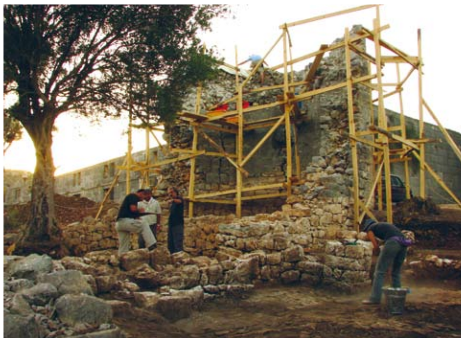
BELOW Excavations underway at Andriake: revealing the first known synagogue in this part of the Mediterranean.
